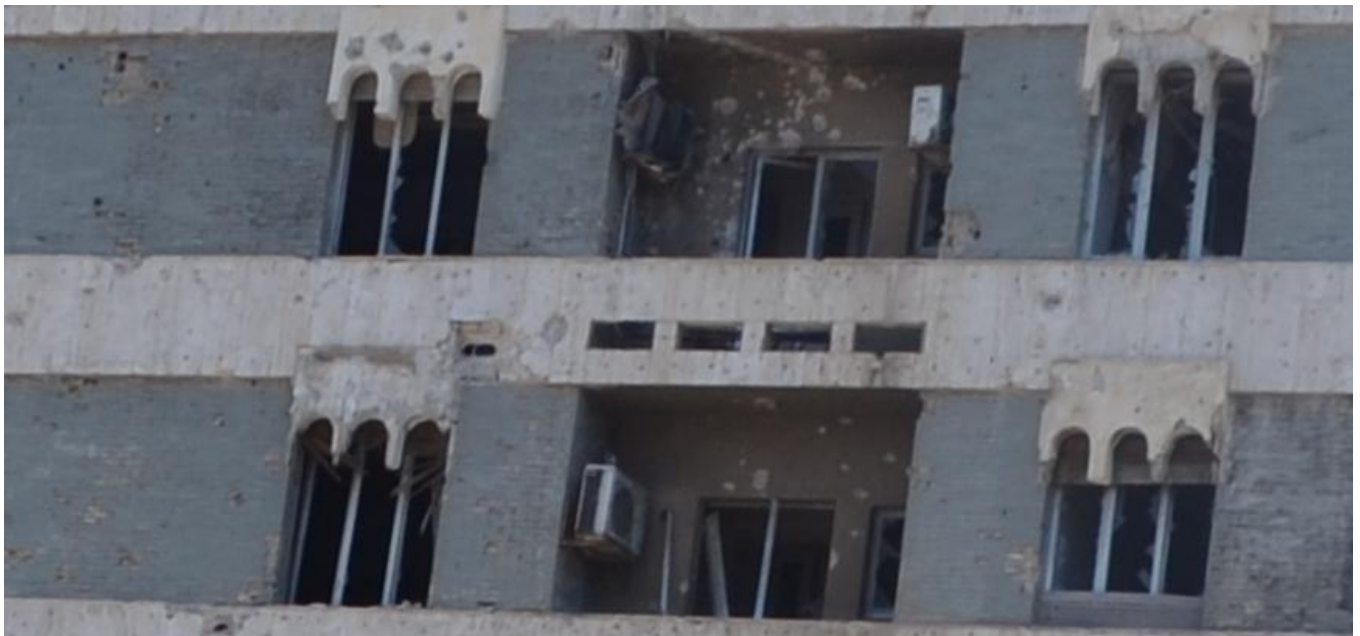
Roof : unknown Walls : Minor damages Doors/windows: severe damages
