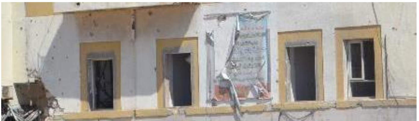
Roof : unknown Walls : Minor damages (just a few bullet holes) Doors/windows: severe damages (all glasses are broken, 3/4 windows are destroyed..)
