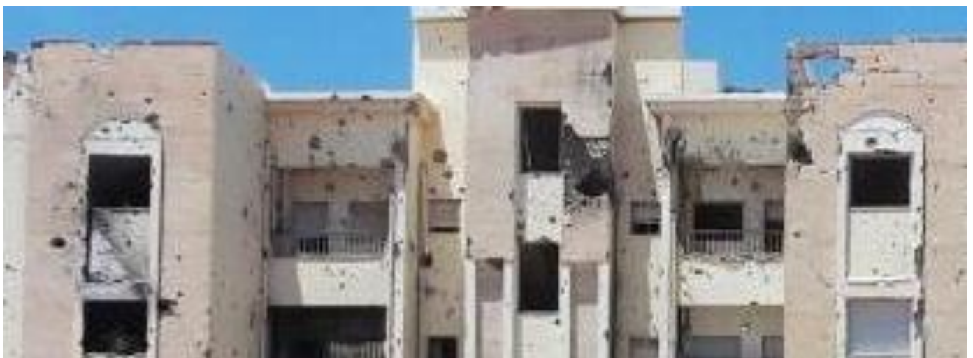
Roof : unknown Walls : Severe damages (many holes, some are large) Doors/windows: severe damages (Most of windows are destroyed.)
