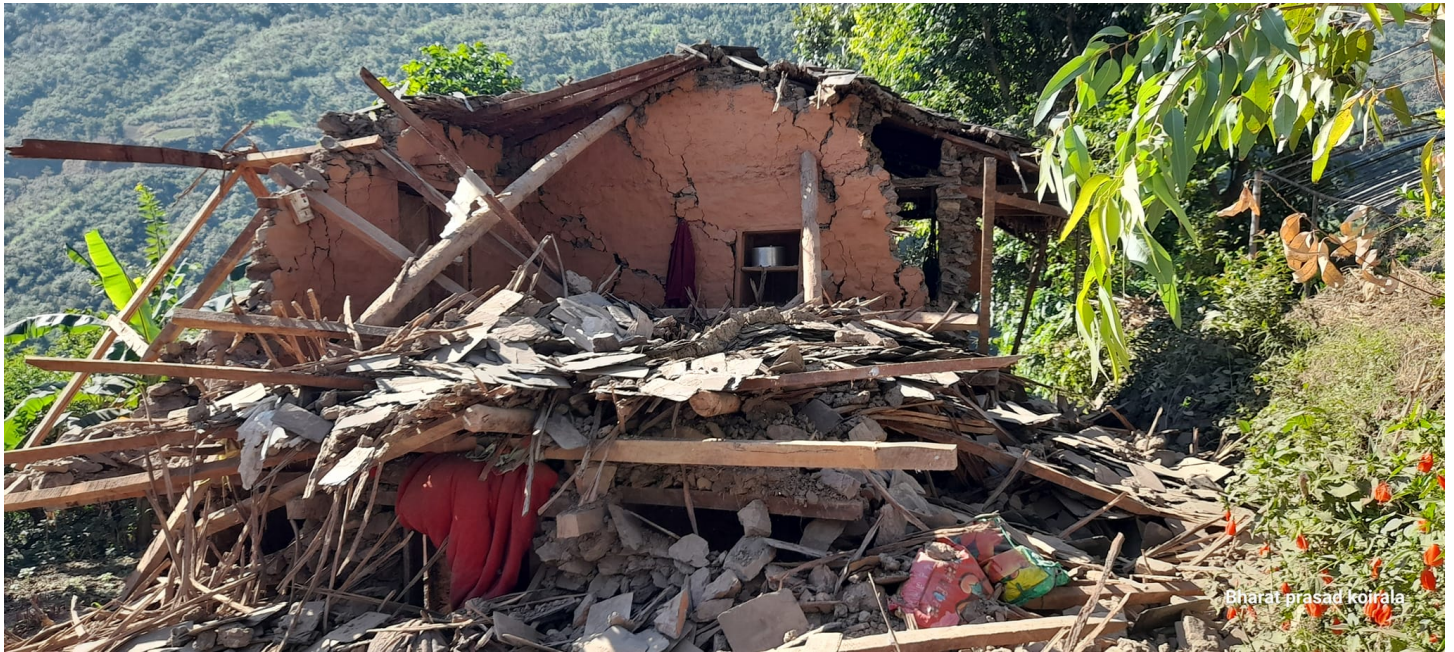
A house destroyed due to the earthquake of 3 November 2023 in Jajarkot District. (Photo: Bharat Koirala, NRCS)
