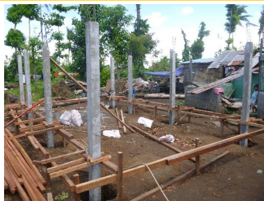
Figure 2: Reinforced concrete columns have been erected for this core shelter in Tabontabon, Leyte. Credit: Philippines Red Cross Haiyan Shelter Programme (Photo W. Eastwood)
