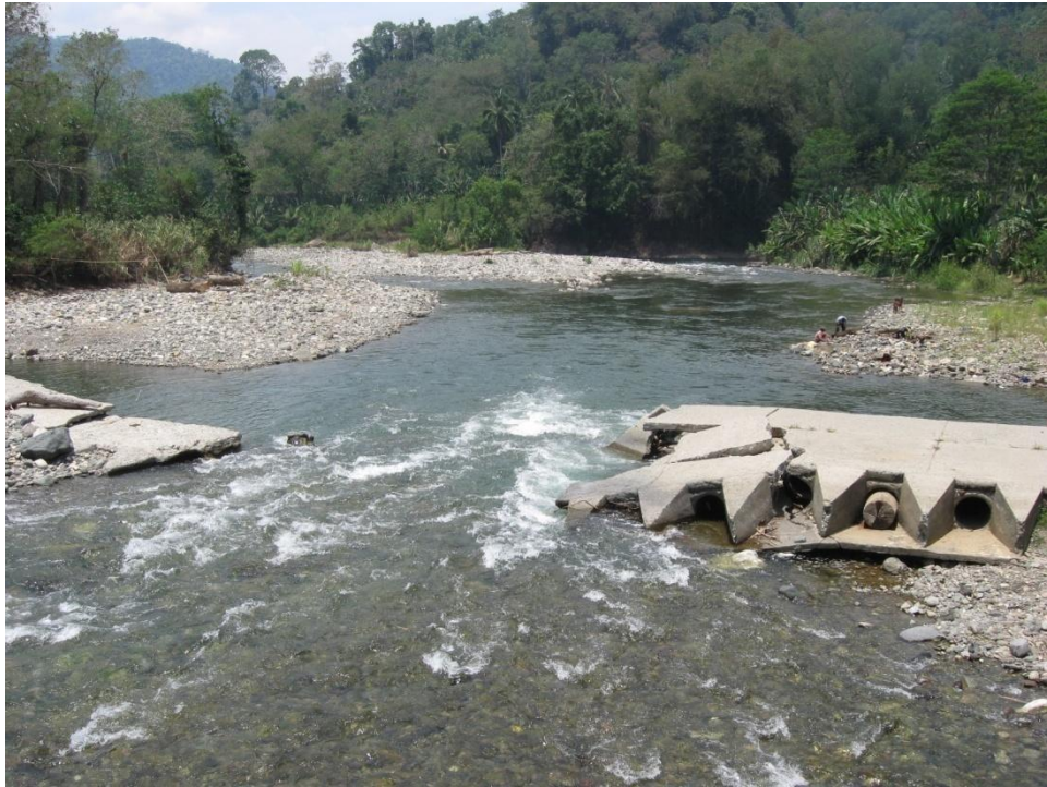
Photo 19. The submarine bridge across Bayug River along the boundary of Purok Kiambong, Brgy. Rogongon and Purok Kadiis, Brgy. Panoroganan was slightly damaged in a 2005 flood and was eventually destroyed by floods in 2009.
