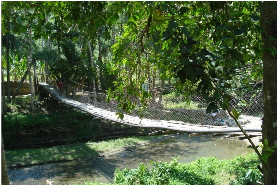
Photo 12. The hanging bridge across Pugaan River in Purok 1B, Brgy. Pugaan was destroyed by flashfloods on May 18, 2009. It has since been repaired.
