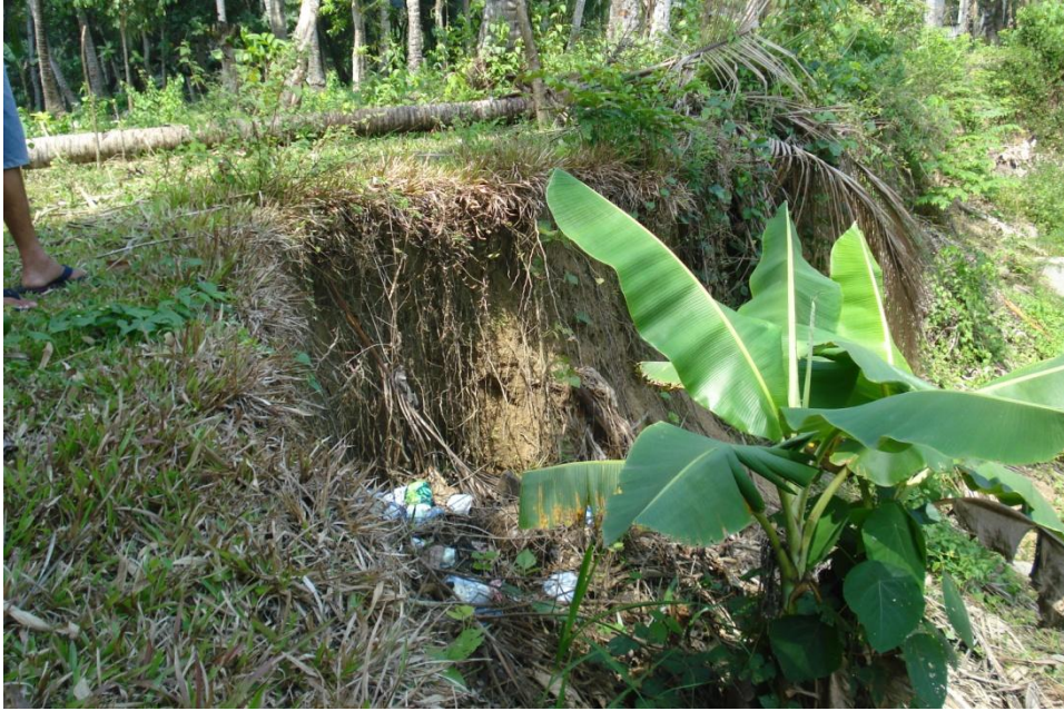
Photo 3. Riverbank erosion was observed along Iligan River in Isla Verde Village, Zone 4, Brgy. Abuno.
