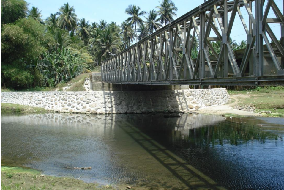
Photo 15. The Tulay ng Pangulo in Purok 8, Brgy. Tipanoy was damaged during the January 2009 flooding event. Riprap structures have since been constructed to protect the base of the bridge from scouring.
