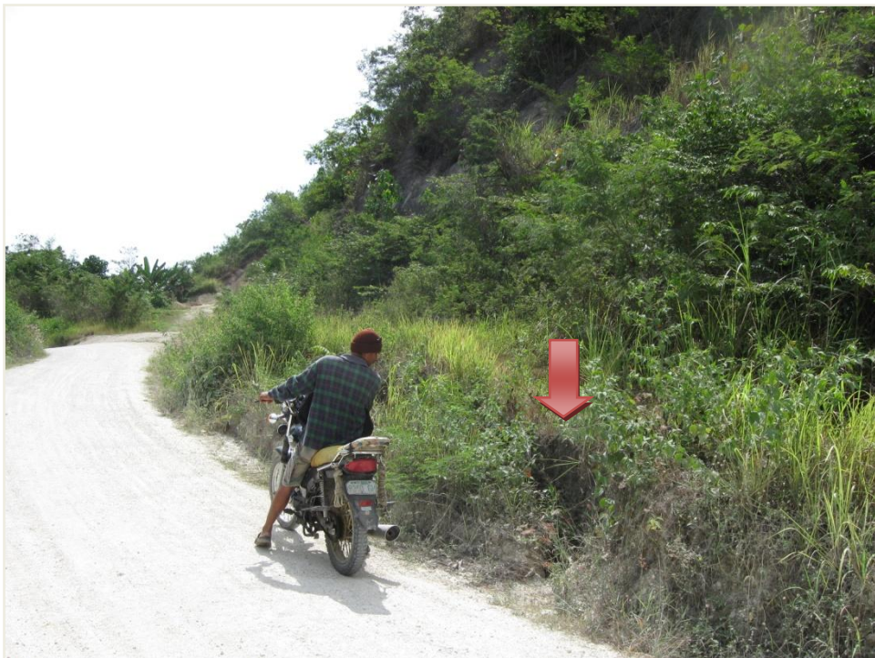
Photo 22. A large crack was observed along the road in Purok 5 Lerop, Brgy. Kiwalan. The crack is reportedly 175 meters long with an average vertical and horizontal displacement of about 0.7 meters and 0.3 meters, respectively. The red arrow indicates one end of the crack.
