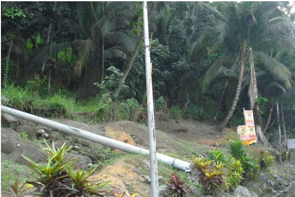
Photo 4. Ground creep was observed along the highway in Brgy. Buru-un as evidenced by bent coconut trees.
