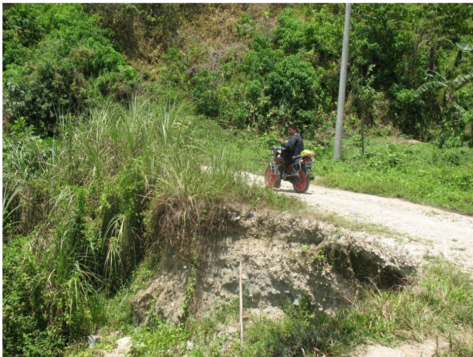
Photo 20. This section of the road in Purok 10, Brgy. Lanipao is prone to landslides.
