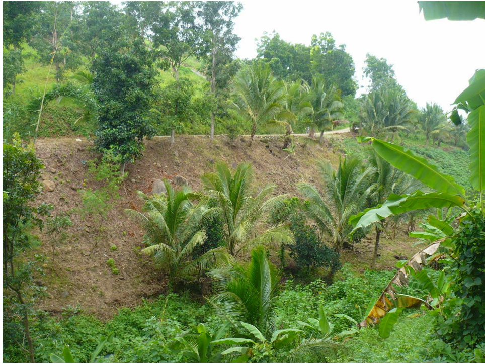
Unstable slopes along the road to Brgy. Balubal as manifested by the tilted coconut trees
