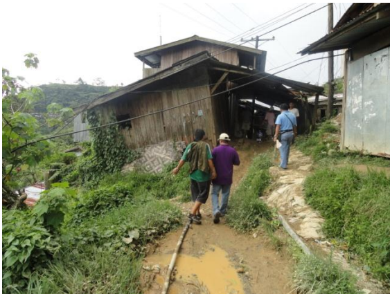
Photo 3. Tilted houses erected at the edge of steep slopes prevalent in Brgy. Mt. Diwata
