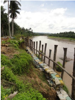
Photo 7. River bank protection against active river scouring located at Brgy. Inambatan
