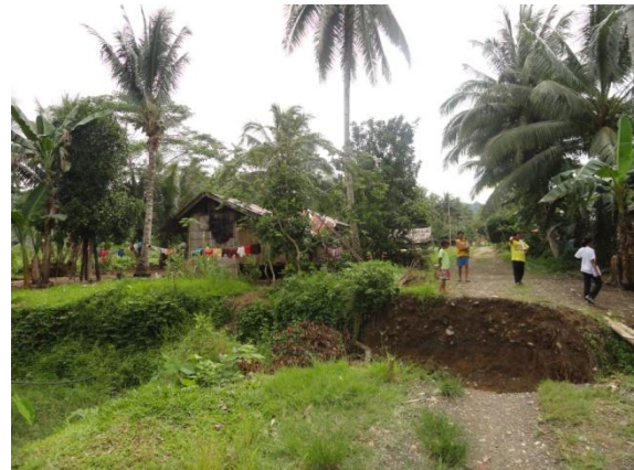
Photo 10. Destroyed culverts in Po. 3, Brgy. Haguimitan due to high stream discharge
