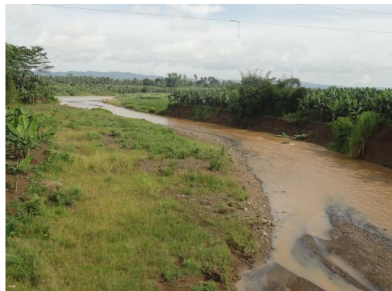
Photo 6. Active riverbank erosion of Mamonga River
