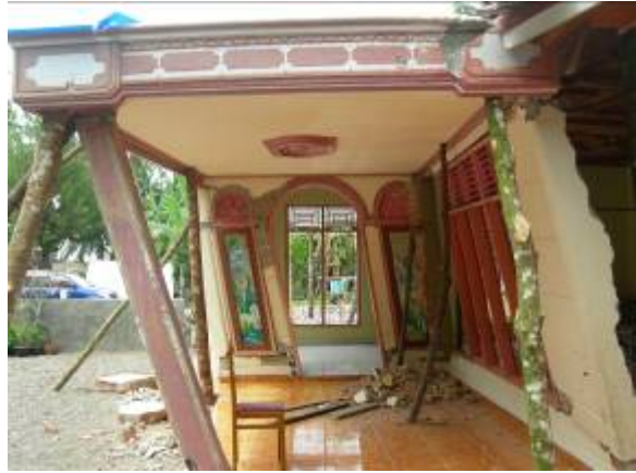
Lack of lateral bracing, dangerous structure.
