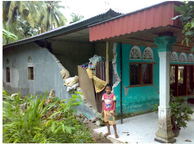
Photo: Beneficiary’s damaged house pre-reconstruction
