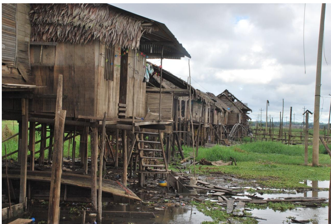
Figure 1: Typical flood damage experienced in the semi-urban neighbourhoods in Punchana, Iquitos
