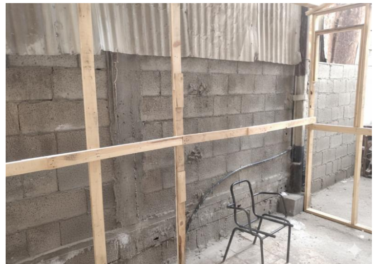
ESK framing built by joining wooden pallet members. The shelters will be tested, and lessons will be shared at upcoming SC meetings.
