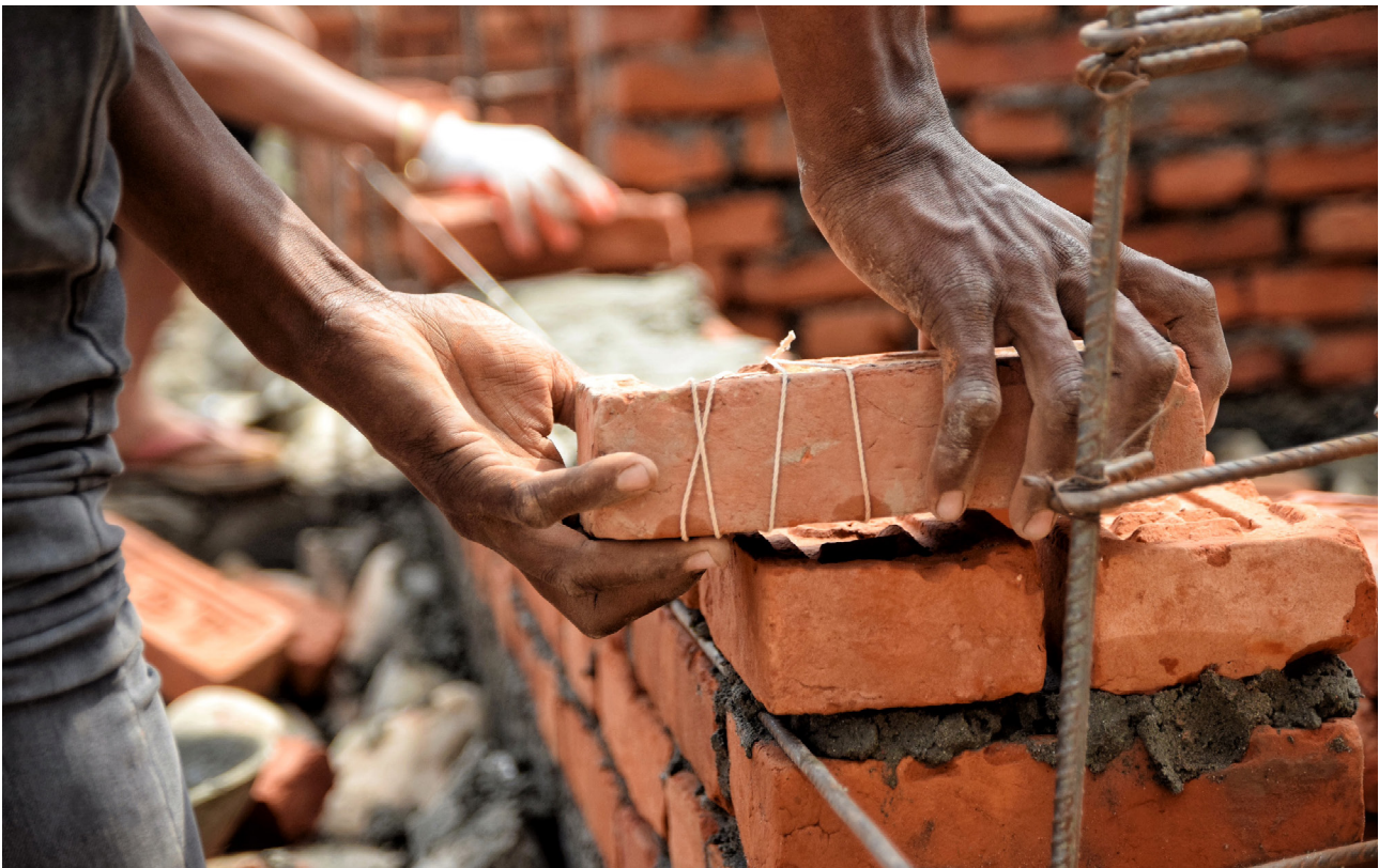
Fig. 2: © Bria Fast. Nepal, 2016. A mason lays bricks during reconstruction of a home after the Nepal earthquake.
