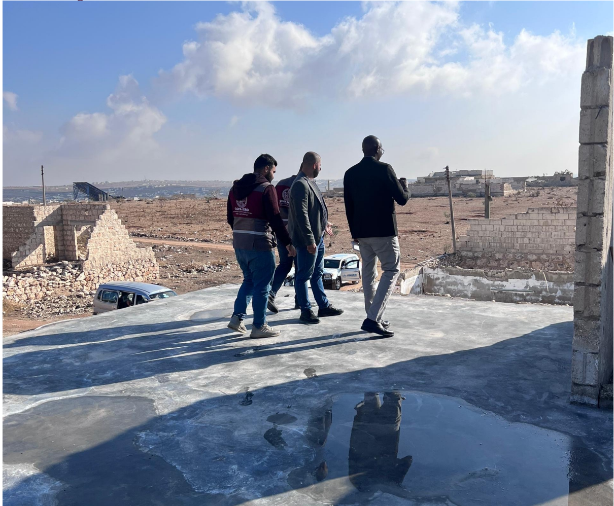
Photo 4: Technical visit to a GOPA-led house rehabilitation site in Ma'arrat al-Numan, conducted jointly with municipality representatives
