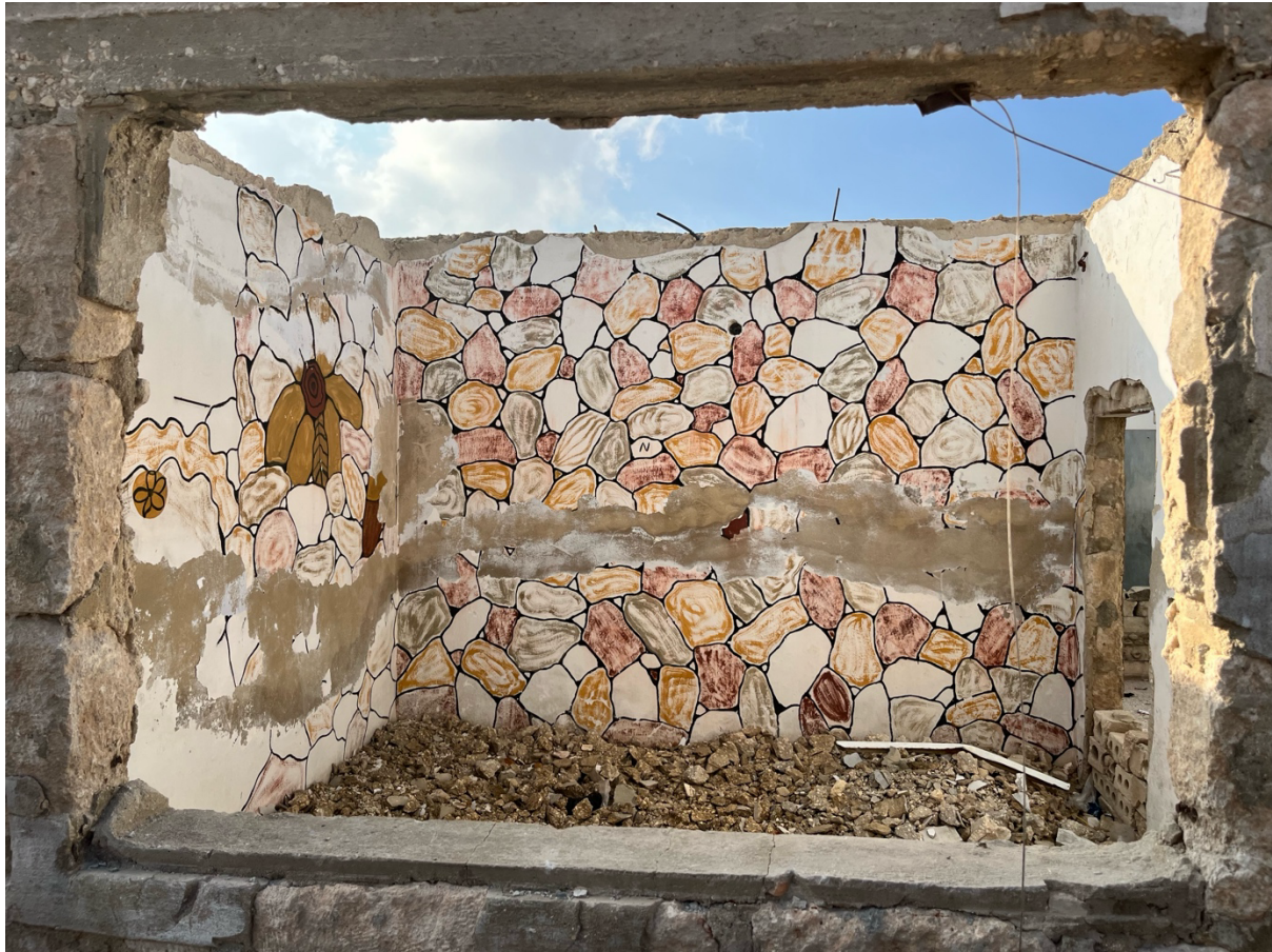
Photo 1: Residential unit in Ma'arrat al-Numan showing complete roof collapse and without windows and doors, rendering the structure uninhabitable.
