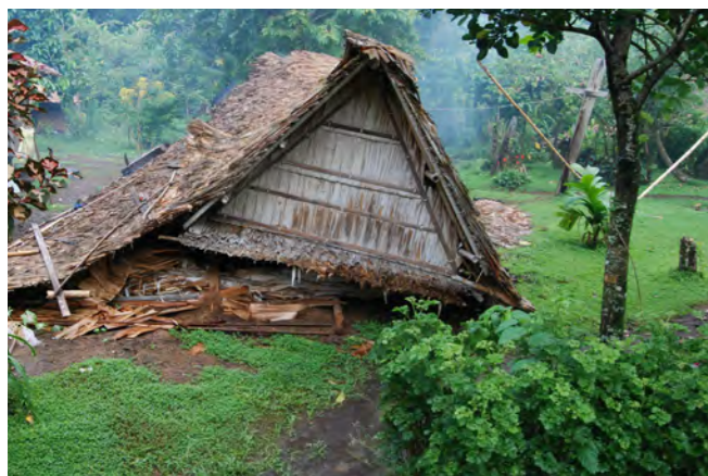
Figure 74: Complete collapse of house but relatively intact roof. (Photo credit: Kaunitz Yeung Architecture)
