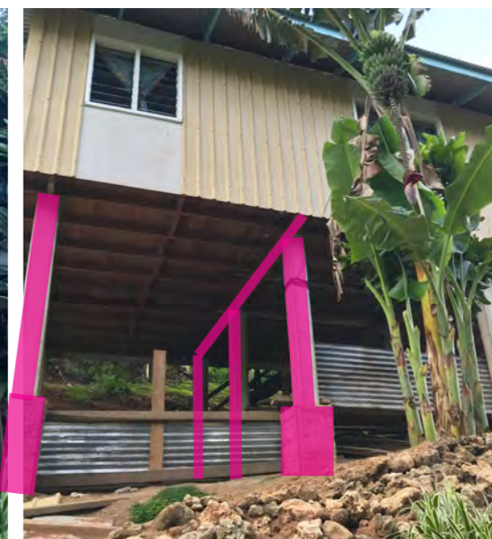
Figure 39: Photo of a house with reinforced concrete stepped footing and reinforced concrete column. Location: Aekafo-Feraladoa settlement (Photo credit: John Clemo)
