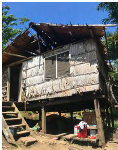
Figure 73: Roof damage due to inadequate bracing, Wind Valley settlement. (Photo credit: John Clemo)
