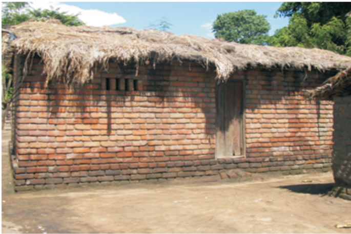
Photo 1 Rising and flowing water causing dampness and weakening foundations
