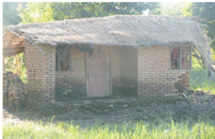
Photo 2 In extreme cases the stability of the house is compromised
