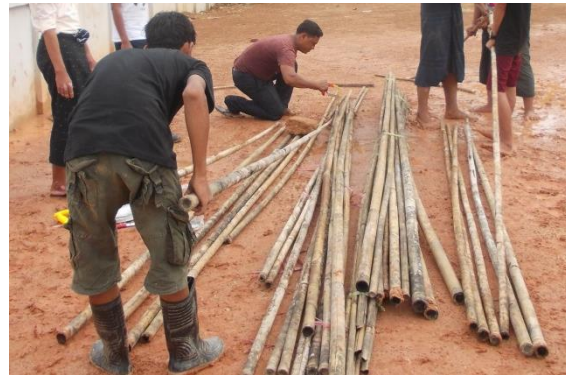
Frame poles. Under specification but adequate.
