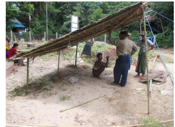
Guy ropes would not be needed if posts are dug into ground
