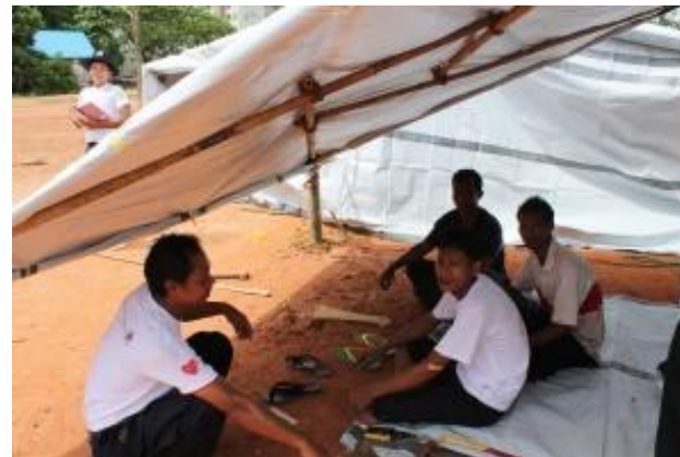
Even a 2 foot elevation makes a considerable difference to living space.
