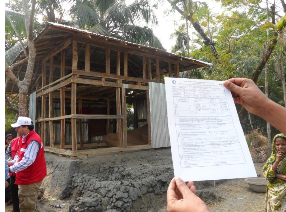
Photo B: Shelter construction is going on in Sadar upazila, Barguna District
