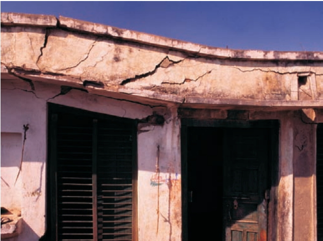
Foundation Settlement due to rising ground water level
