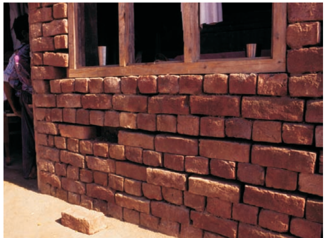
Scouring of mud mortar from open joints by fast moving water
