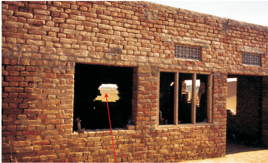
Damage to rear wall by suction
