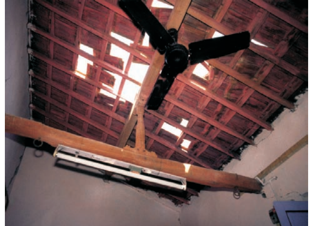
Roof Tiles blown off
