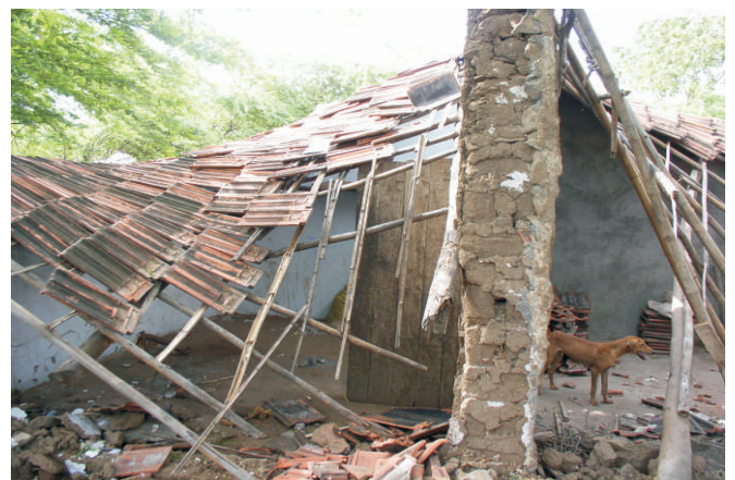
Wall & Roof damage by Cyclone
