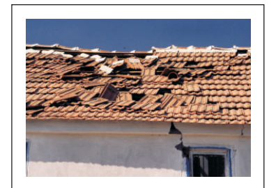
Roof distortion damage
