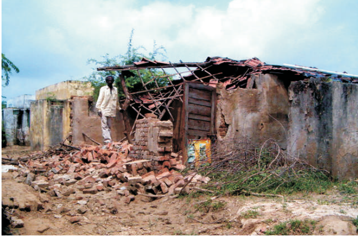
Collapse of wall and damage to roof
