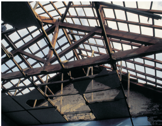
Blown off tiles due to high winds
