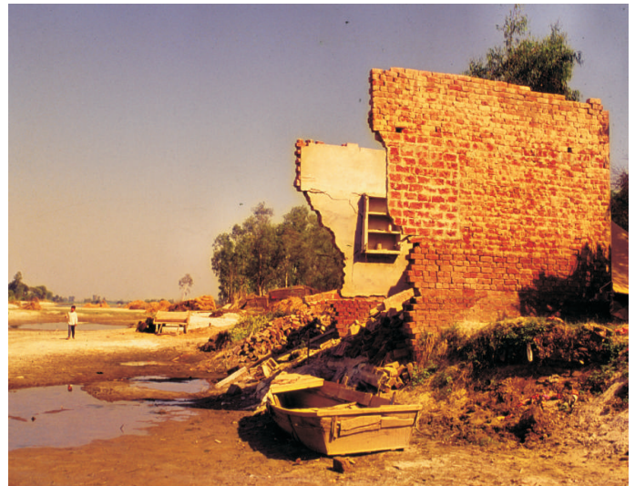
Wall collapse due to tidal surge
