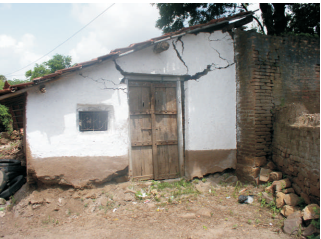
Scouring of wall base & cracked wall
