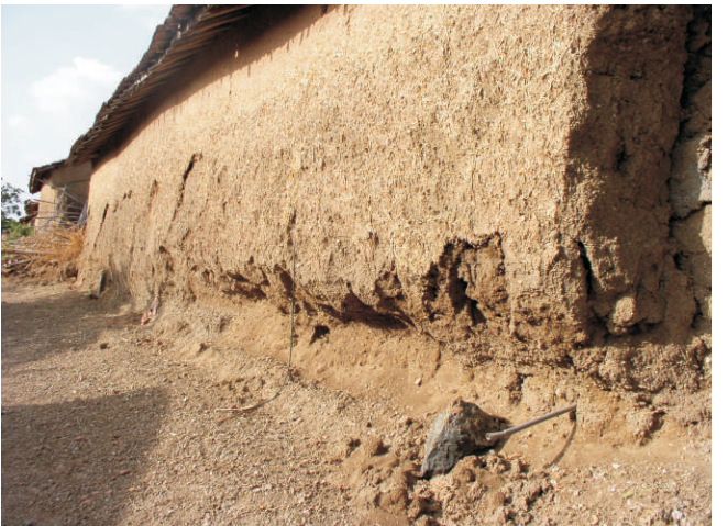
Erosion and scouring of mud wall by heavy rain
