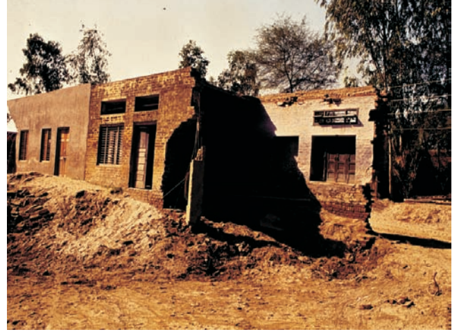
Collapse of wall due to mud mortar weakening
