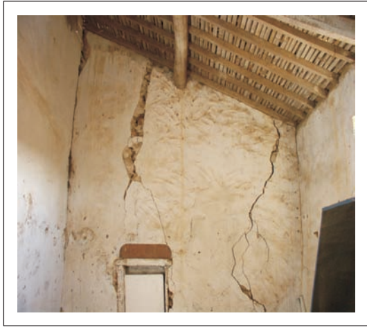
Moderate and fine cracks
