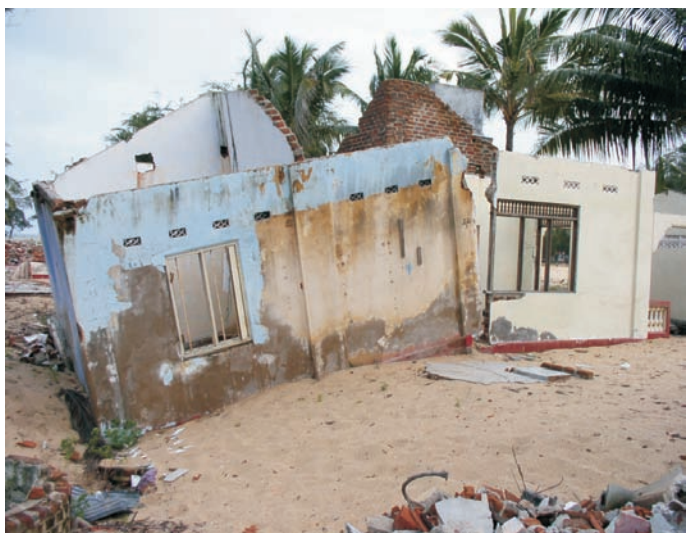
Damage due to foundation settlement
