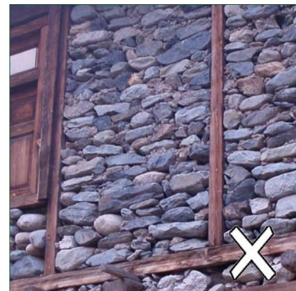
Stonework with no bracing.
