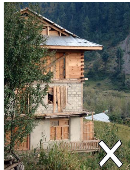
Building height greater than length or width.
