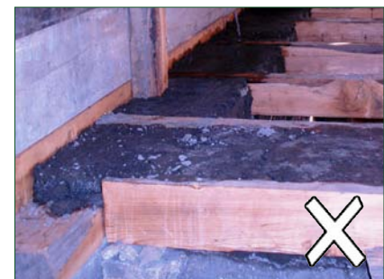
Heavy insulation in the roof is dangerous.
