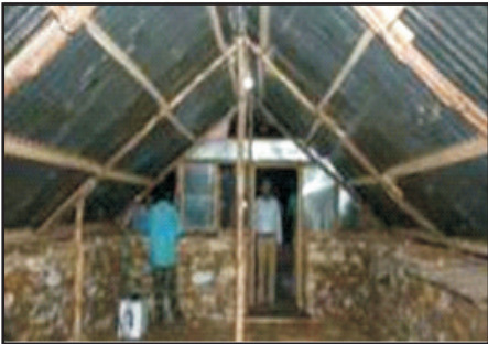
The interior space is large where a person can stand up even near the wall.
