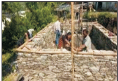
Connect the wall plate to the vertical posts in gable walls using metal strap and nails.
