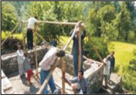
Attach rafters to ridge beam and wall plate with GI strip and nails.
