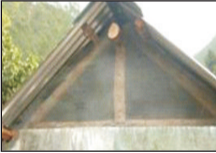
The triangular portions in the end walls above the lintel level should be covered with metal mosquito netting to permit lighting and ventilation.
