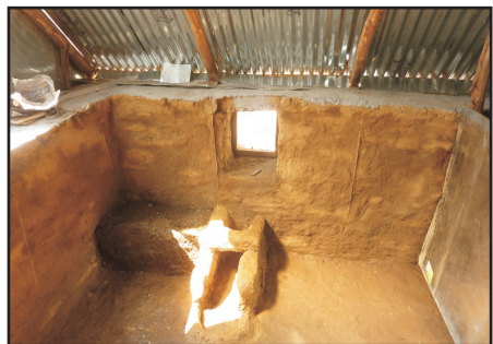
Finished interior with a window, wood burning stove and storage space above the finished wall.
