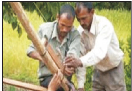
While installing these on top of ballis use packing under purlins to compensate for the unevenness of the ballis.
