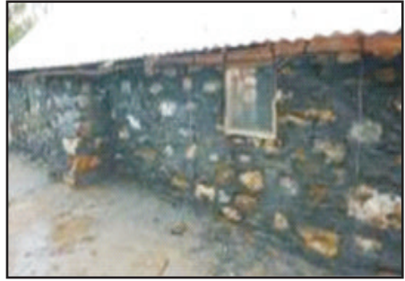
Side view with small window and butress with acts as a smoke vent in a kitchen. A butress is to stabilize the long wall against earthquake forces.
