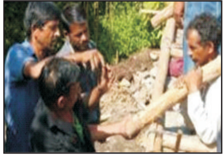
Always use hand drill for making pilot hole in all timber joints
