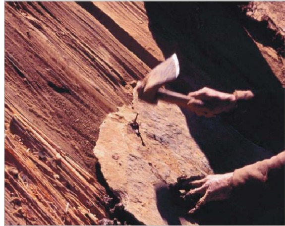
Slate tiles to be anchored to roof planks with two minimum two nails.
