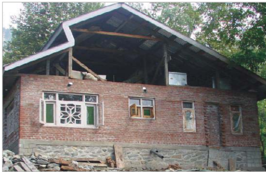
Material can be changed at a particular height, like stone in the plinth, and brick in the walls.
