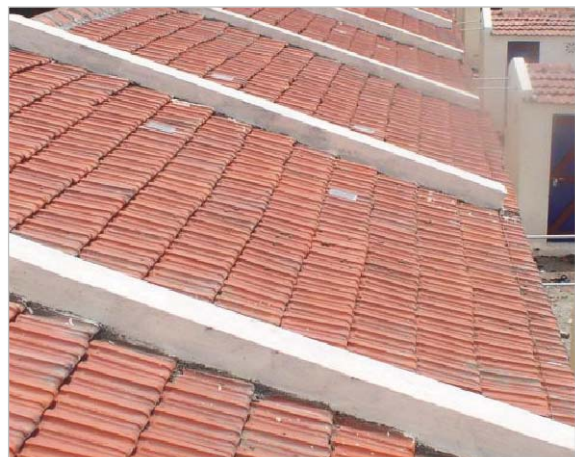
Construct narrow load walls over clay tile roofing at 4' (1.2m) spacing in high wind-speed areas .
