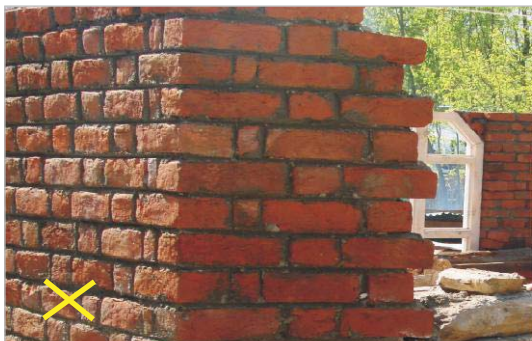
Wall-to-wall connections: Toothings left projecting out at the end of a wall result in weak joint with another wall.
