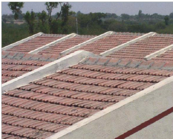
All ridge tiles must be installed using cement mortar, especially in high wind speed areas.
