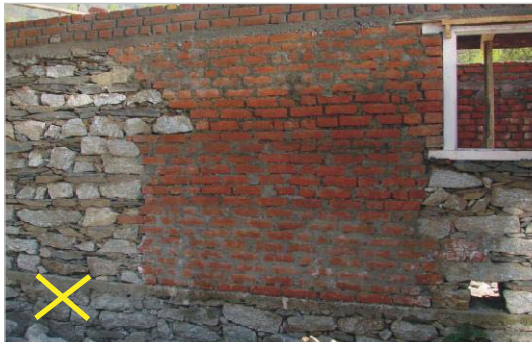
Do not use different materials side-by-side or next to each other in a structure.
