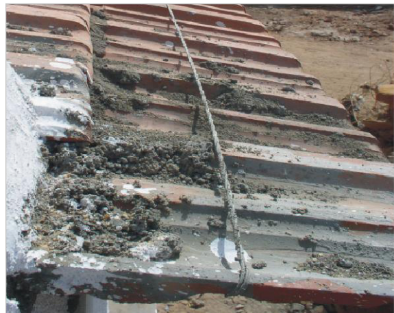
Install steel rod or GI wires on the bottom-most row of clay tiles.
