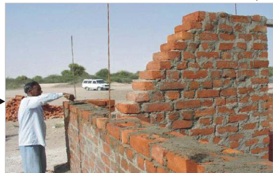
Build all the walls at the same time. Or else, leave the end of a wall in stepped manner to later connect it with another wall.
