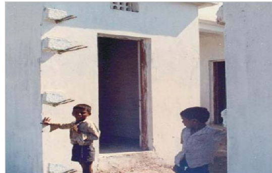
The joint between the old and the new construction must be done with bars embedded in old wall to ensure disaster safety.
