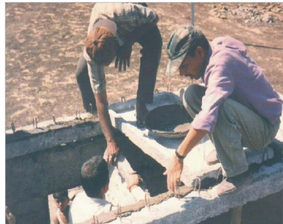
Flat stone or pre-cast doubly curved concrete panels supported on pre-cast RC joists.
