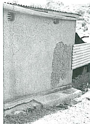
This is an attempt to build foundations after the wall had been built
