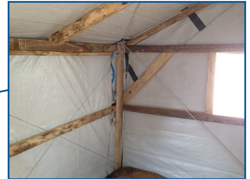
Lateral (wall) bracing can be done with tie wire or rope, if timber is not available.
