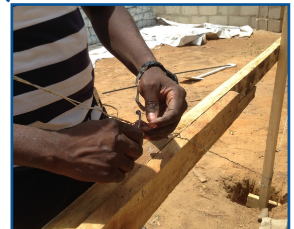
If using tie wire for bracing, twist it in order to tension it well
