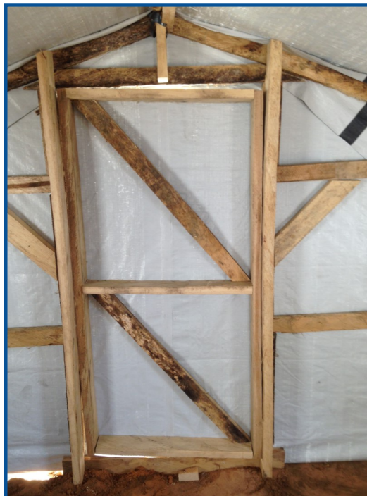
Brace the door and use cut-offs from the timber to brace joints
