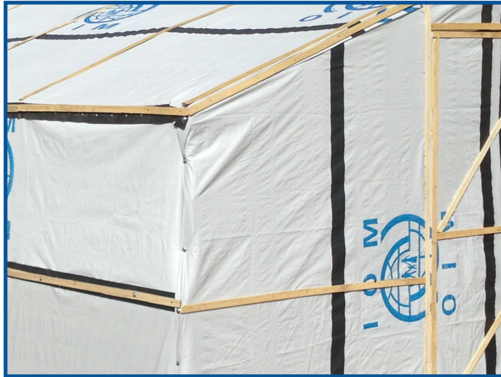
Add battens to ensure that the plastic sheets are pulled tight and do not flap with the wind.
