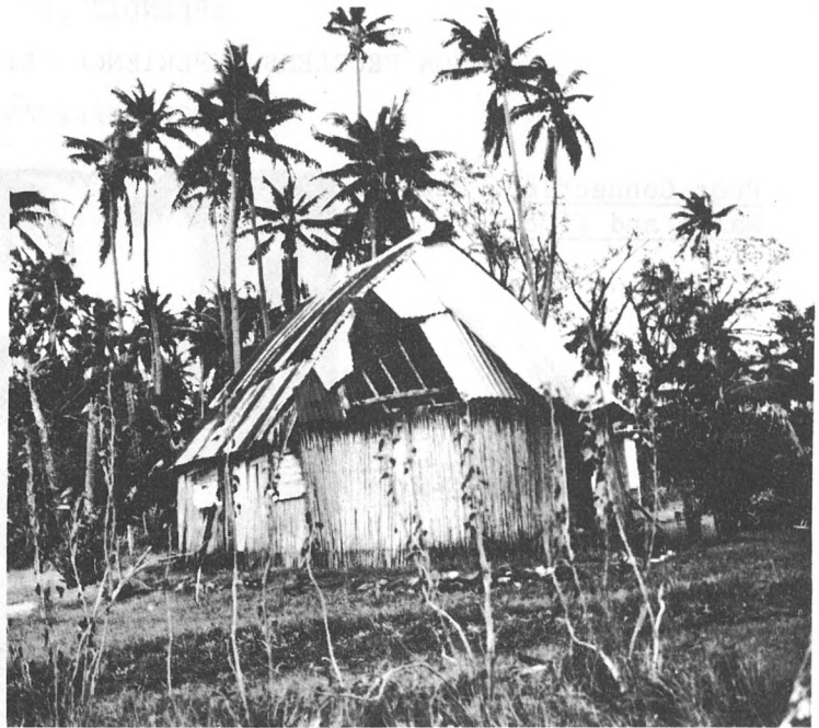
Inadequate Nailing of Corrugated Iron to Purlins
