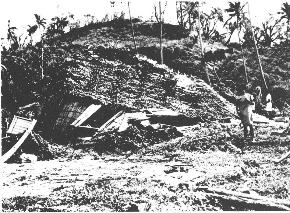
Inadequate Bracing in Walls
