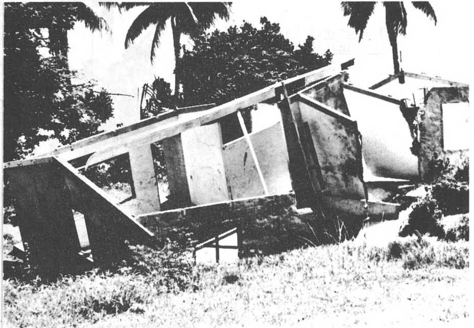
Poor Connections Between Walls and Floor
