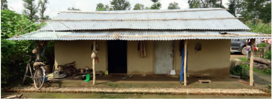
Veranda roof separate from main structure.
