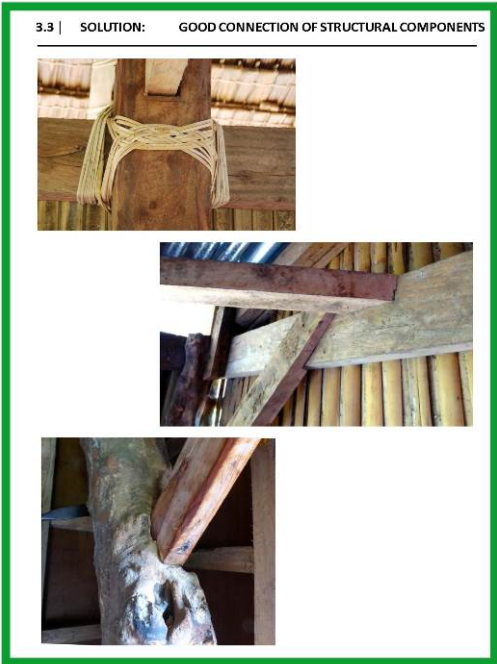
DRR Training – Shelter resilience | M3 - How to increase sturdiness of the building | CRATERra 17
