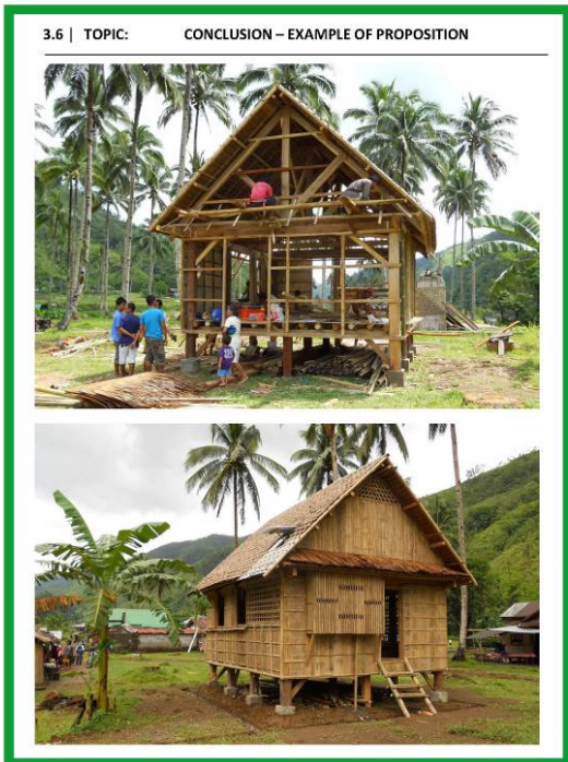
DRR Training – Shelter resilience | M3 - How to increase sturdiness of the building | CRAterre 41
