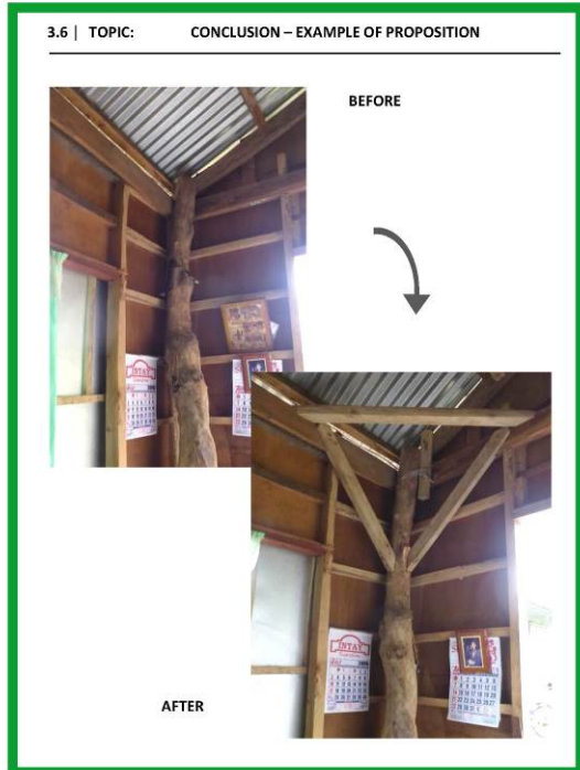
DRR Training – Shelter resilience | M3 - How to increase sturdiness of the building | CRAterre 42
