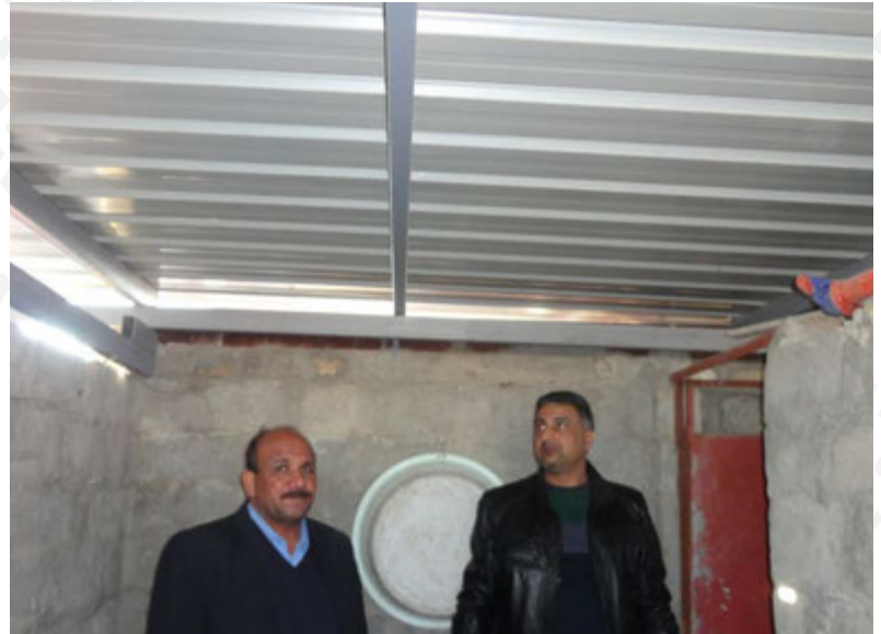
New roof with metal frame and sheet sealed with water proof silicon compound to prevent leaking.
