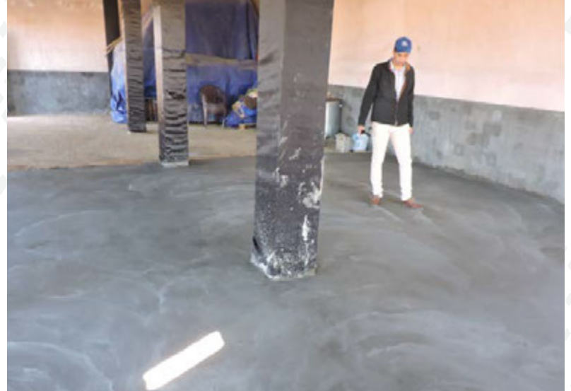
A family's living room floor is rehabilitated with 10cm reinforced concrete floor and structural column.
