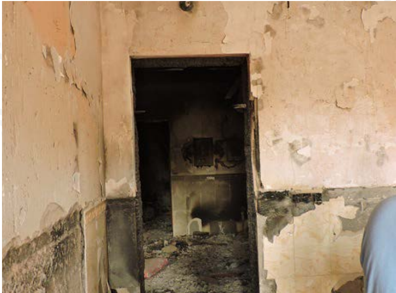
Damaged and burned masonry wall led to an unsuitable living environment.
