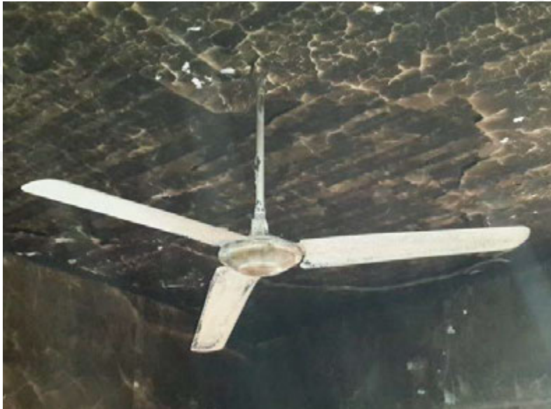
Roof ceiling damaged by fire. Ceiling structure may collapse and is unsafe for living.
