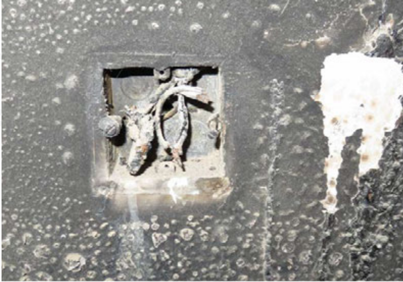
Damaged wall with exposed electricity creates unsafe conditions.
