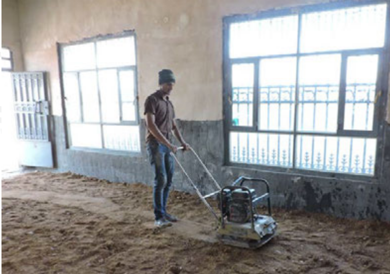
Concrete floor damaged; a new floor is needed.
