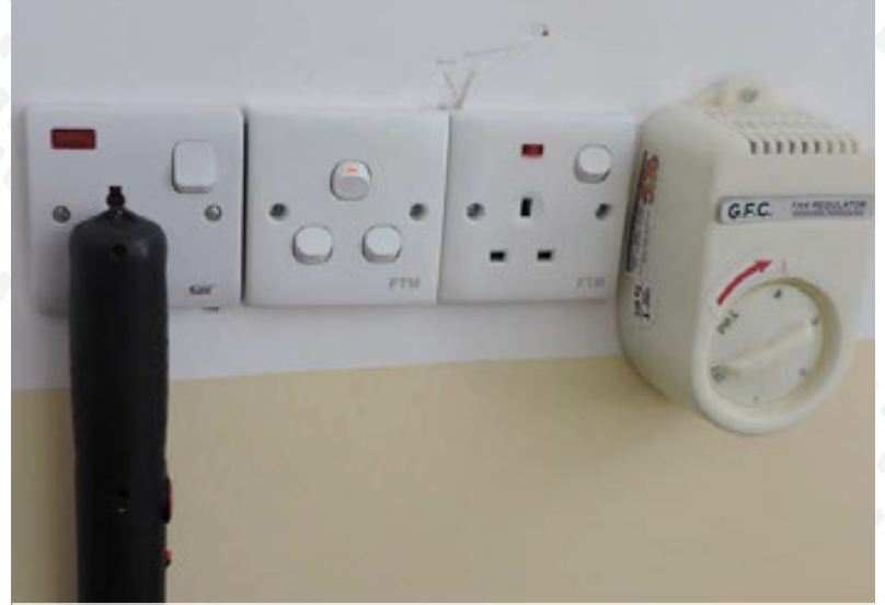
A family's living room is rehabilitated with new electrical wiring, light fixtures, and electrical earth grounding.
