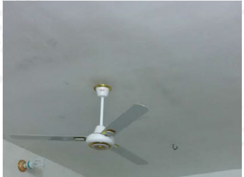
Roof ceiling rehabilitated: roof frame replaced with cement plaster; new painting and electrical fixtures.
