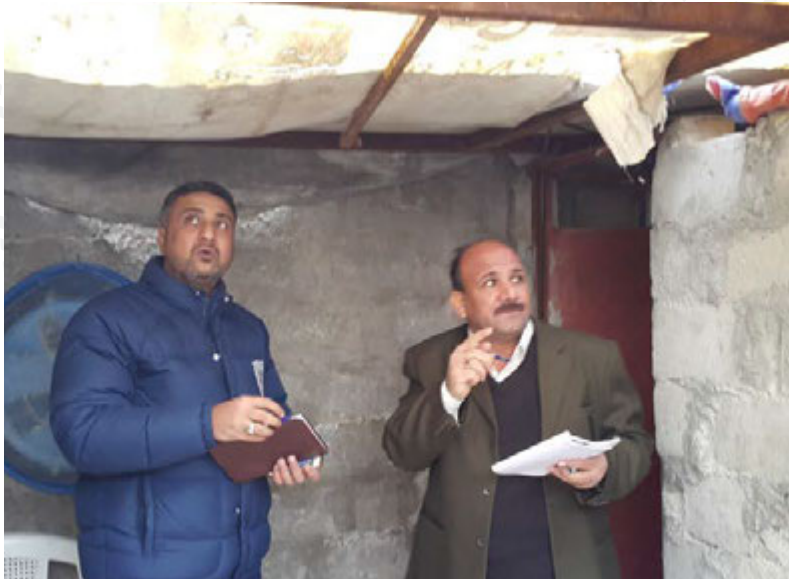
Roof leaking due to the poor quality of the roof support and of roofing sheets and frames.
