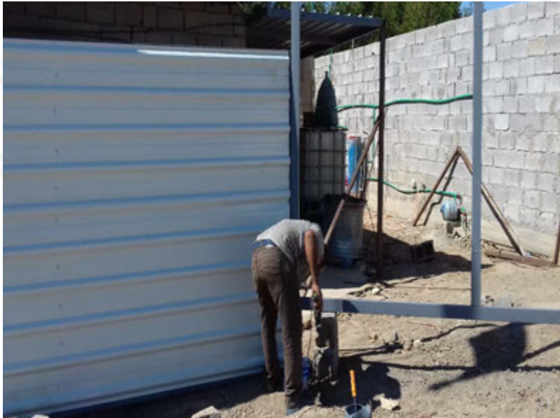
Unprotected shelter, vulnerable to intrusions; lack of privacy.
