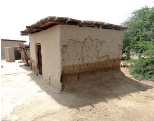
Figure 14: Example of adobe wall in need of repair
