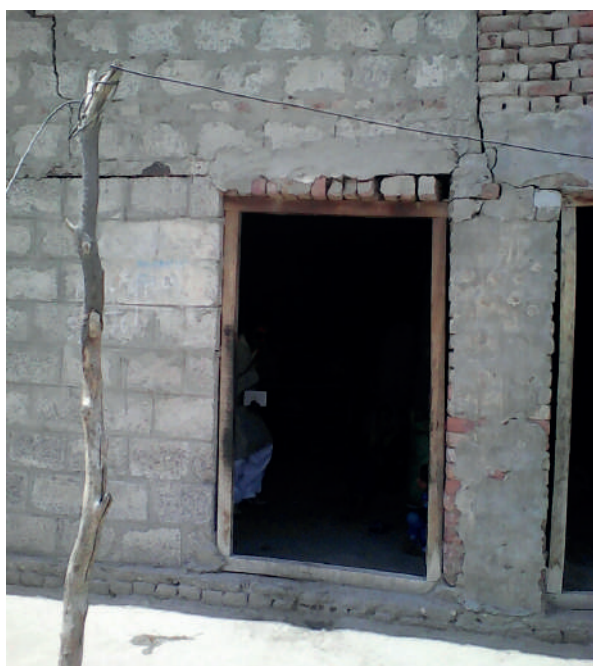
Figure 08: Example of low strength wall
