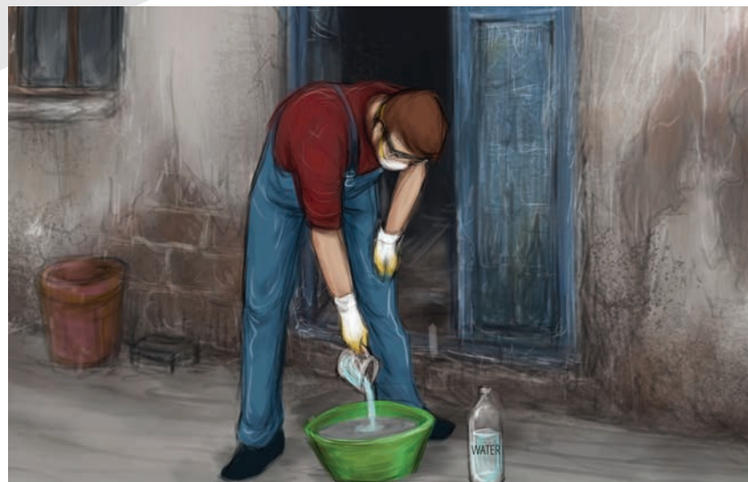
▶ Add water according to the required ratio (5 kilogram mortar to 1 liter water) for the amount of cement mortar needed.
