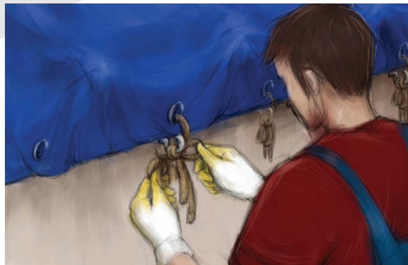
▶ Fasten sides of the plastic sheets to the iron nails that have been mounted to the wall using the ropes.
