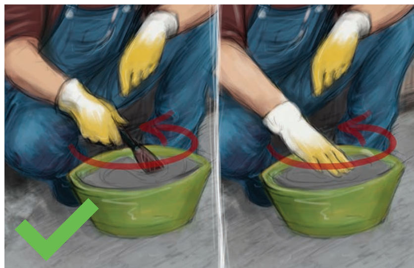
▶ Mix it well using a trowel or by hand until the consistency is semi-liquid and without lumps.
