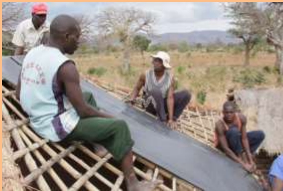
Plastic membrane fitted prior to thatch providing additional protection especially at times when there is a shortage of thatching material.
