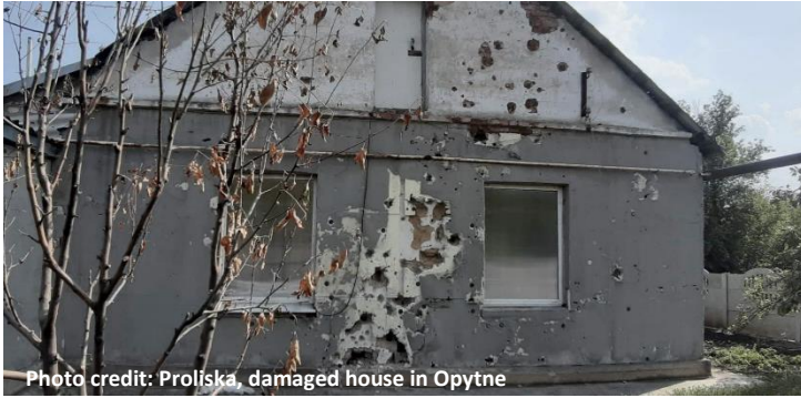
Photo credit: Proliska, damaged house in Opytne
