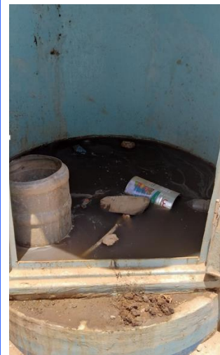
Filled up toilet with an overflow with floating tins at Amman Bin Yasser Collective Centered.
