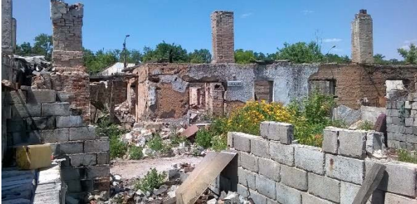
Figure 1-Category 4 damaged homes along contact where vulnerable and elderly still reside as they have no other housing solutions. Credit: A. Meyer
