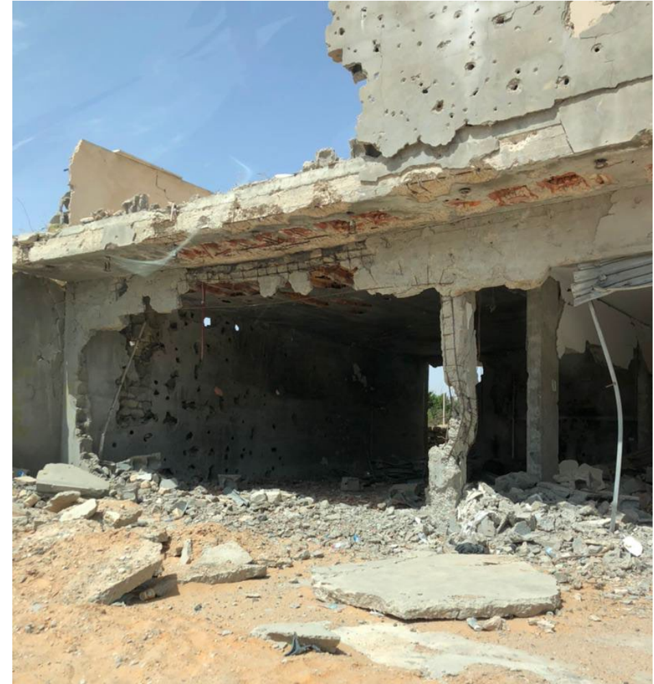
A house damaged by the conflict in Abu Salim, Tripoli
