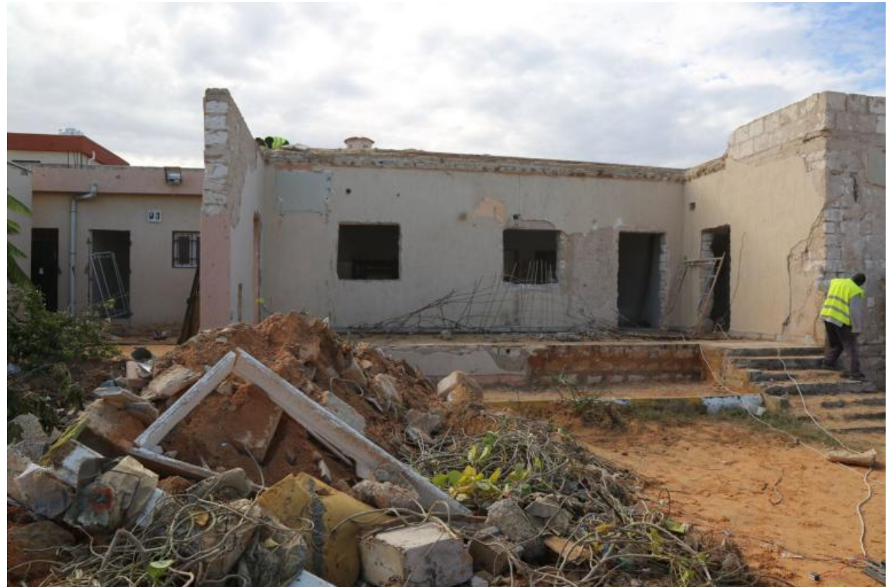
A damaged medical centre before it was rehabilitated by NRC
