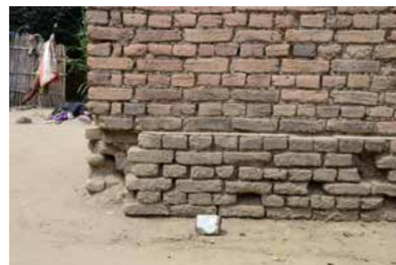
8. Absence of protection at the wall base towards water erosion.
