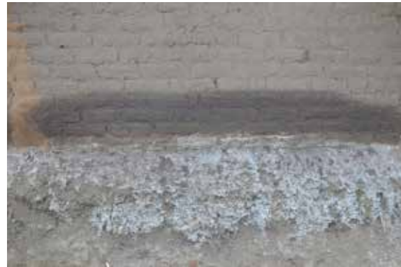
1. Absence of damp proof course. Moisture reduces wall resistance
