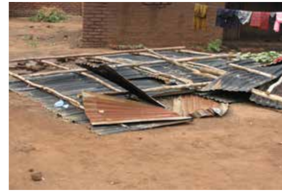
9. Blown off roof
