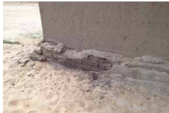
3. Erosion of the foundation. Protection with cement is required
