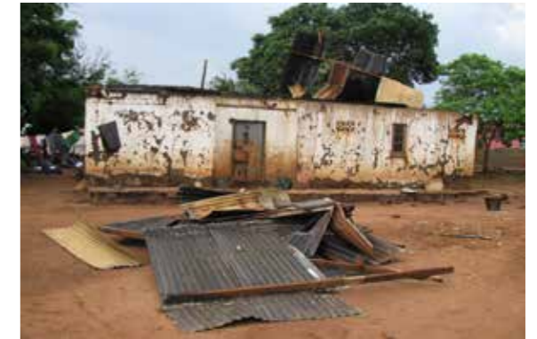
10. Blown off roof
