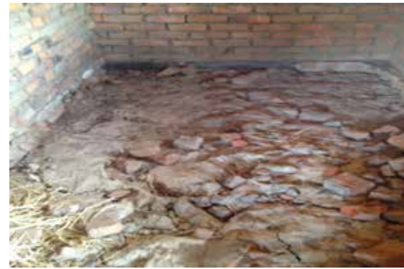
2. Mud pavement erosion due to water exposition
