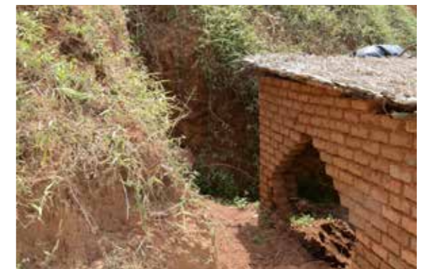
14. Wall collapse after landslide
