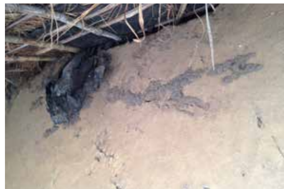
5. Termites reaching the wood structure of the roof
