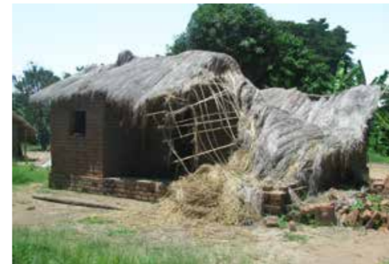
11. House collapsed because of the earthquake
