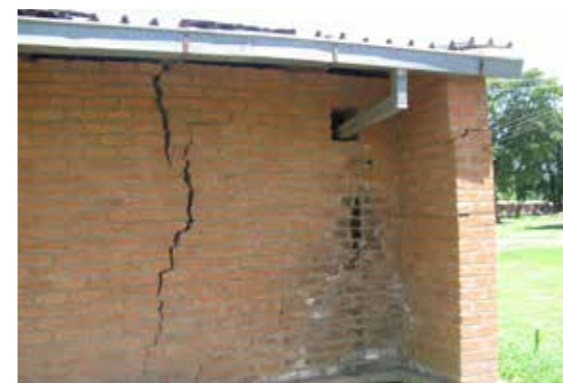
15. Cracks damage the wall because of the earthquake
