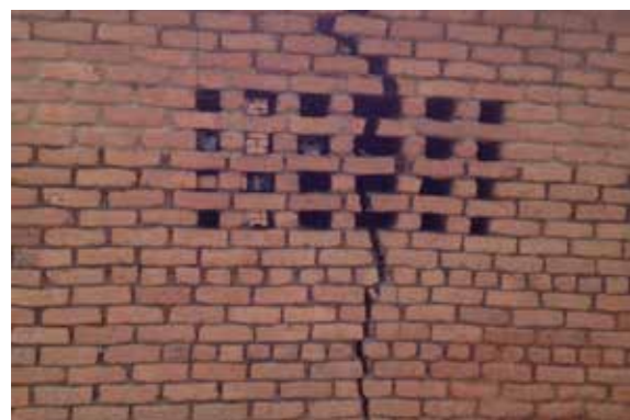
7. Cracks damage the wall because of the earthquake
