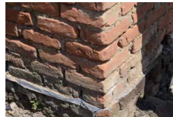
13. Poor damp proof membrane – exposed wall base to water
