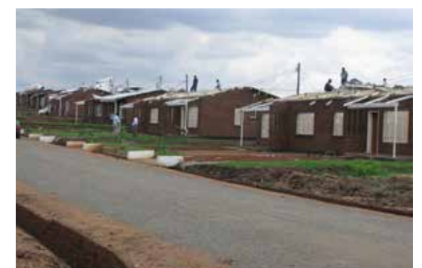
16. Blown off roof
