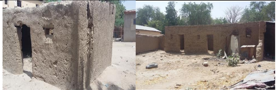
Showing typical damage situation that warrants light repair of category 3
