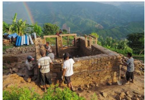
The photo on the left shows the Sunar family members and the masons from the community who constructed the house. The young man in the center with the brown shirt is Ram Sunar, who will live in the house.
