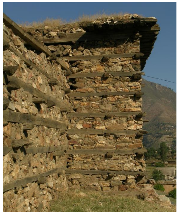
A 19 th century timber-laced rubble stone fort in Northern Pakistan near epicenter of 2005 earthquake that killed 89,000 people. It survived with very little damage despite having been abandoned and unmaintained for half a century! (Photo by author)
