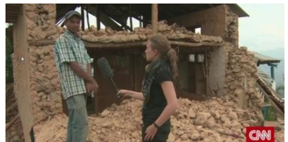
Collapsed house showing horizontally bedded rubble stone construction in Gorkha District. (web)
