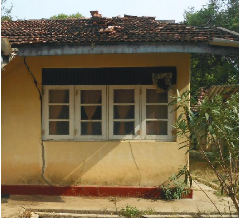
Image: 1a. Vertical Crack along the Wall
