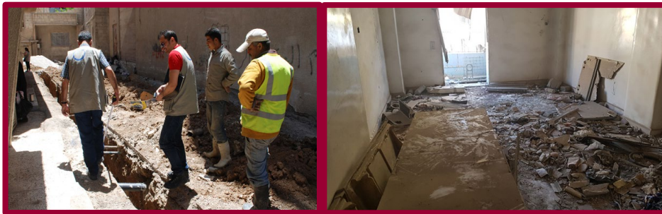
Rehabilitation of partially damaged apartments in Deir Ba'alba, Homs. September 2021 credit: SIF
