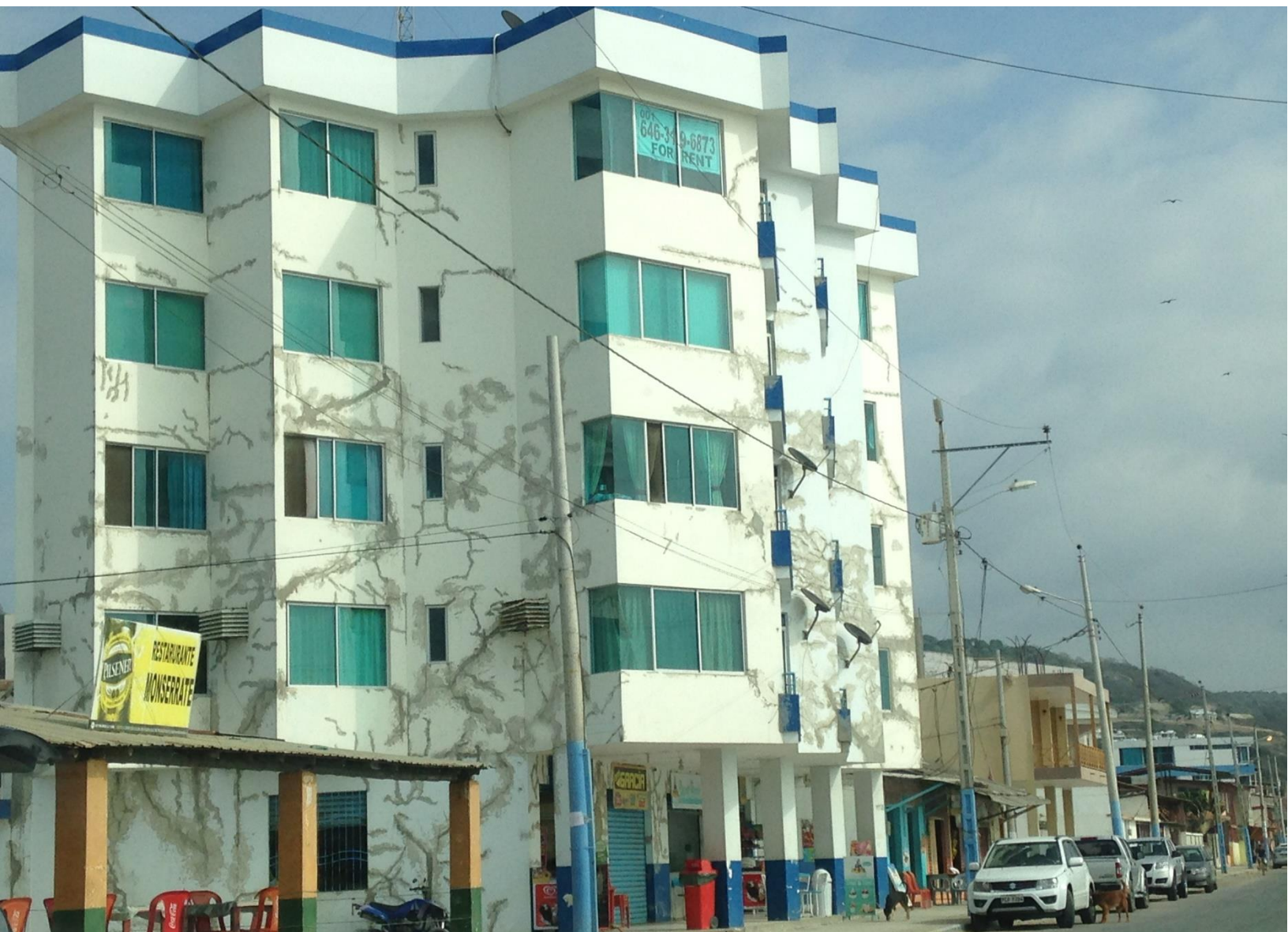
Building in Portoviejo, Ecuador, damaged in the April 2016 earthquake. Taken by Casie Venable.
