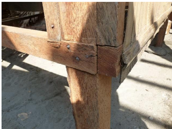
Left: An example of floor beams not extending past the column, and being nailed too close to the end of the piece of coco lumber, causing it to split, consequently losing strength.
