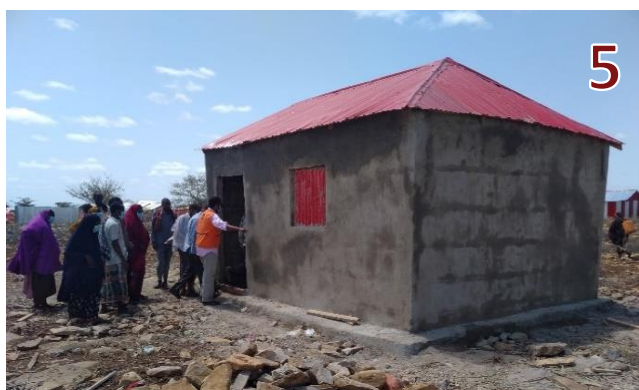
► "Barako 5mx4m" type shelter made up of natural wooden stick walls with stone plinth protection and CGI roofing and verandah. The shelter is plastered with cement/sand mortar on the outside.
