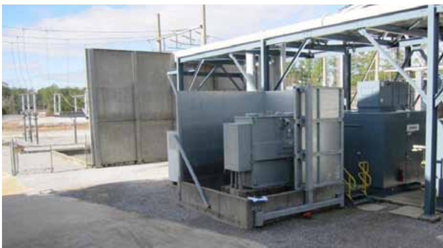
SCS Plant Crist, Florida US.
