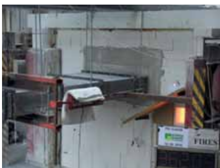
Kitchen Extract Duct
