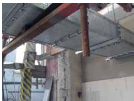
Smoke Outlet Duct
